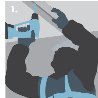
1. After fixing the head track, the floor track should be positioned by using a vertical stud and a laser/spirit level.
